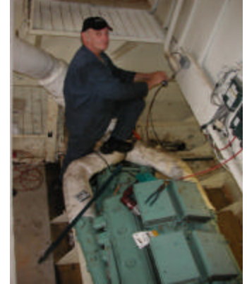
Randy Baygents is hard at work making finishing touches to the engine room.
